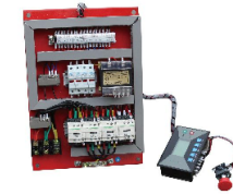
SCREW COMPRESSOR CONTROL PANEL
